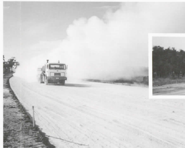
Photographs: Bottom left: work on the project. Above: pavement stabilisation. Above right: duplicating the carriageway, 1987.
