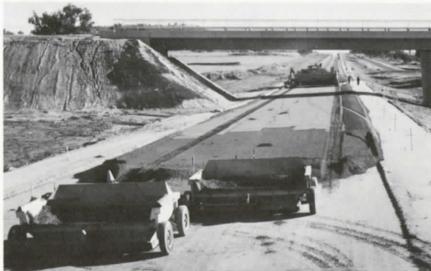
• Above : Construction of the duplicate carriageway at the Murray Valley Highway Interchange • Cover : Bridges over the North East railway at Wodonga
