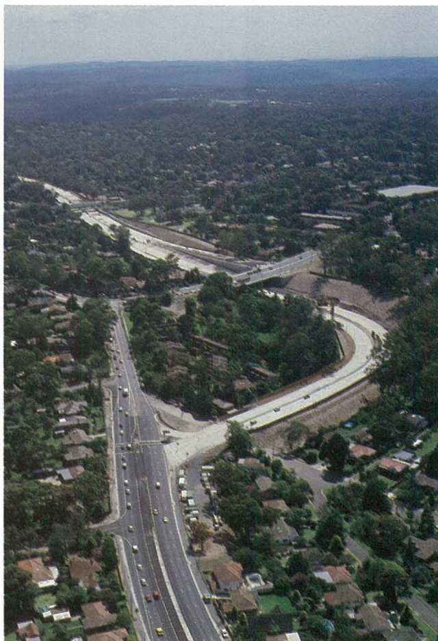
(Above) Work nearing completion on the intersection of Pennant Hills Road, the Pacific Highway and the new section of Freeway at Wahroonga. (Top Right and Below) Asphaltting in progress on the newly-completed Freeway at Berowra.
