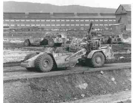
Heavy construction machinery at work at the Tunnel casting basin at Port Kembla
