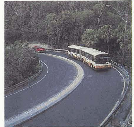
Widening of the bends at Bilgola has allowed the Urban Transit Authority to extend articulated bus services to Palm Beach.
