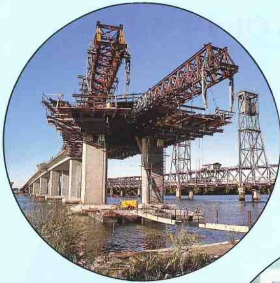
Duplication in progress of the bridge over the Hunter River at Hexham on the Pacific Highway.
