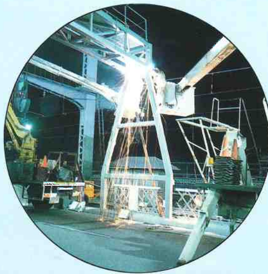
Sparks fly while erecting a gantry for installation of the electronic lane control system, on the Sydney Harbour Bridge.
